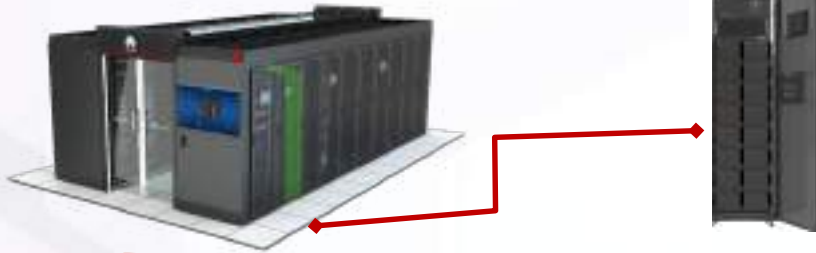
R24 Dual-Row Cabinets with Lithium Batteries Installed in Row
